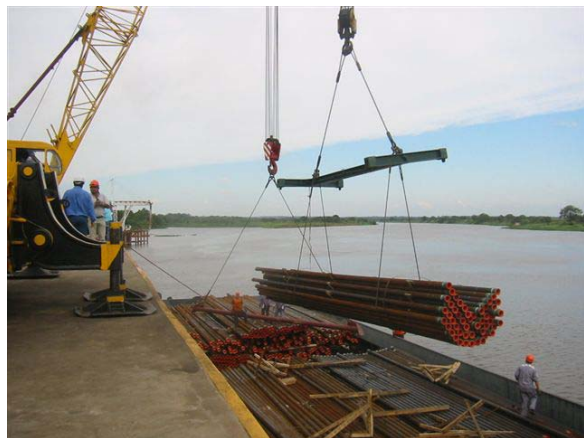
Drill casing being unloaded from barge for loading onto trucks and hauling to the logistics base at La Patria at the end of the paved highway, near the center of the Boqueron Block
