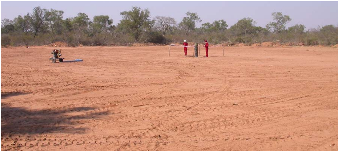
The drill pad cleared and graded, ready for the drill rig and man camp at the Independencia 1 well site on the Gabino Mendoza Block
