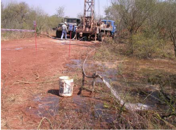
Testing the water well for supplying water to drill the twin well to the Independencia 1 well on the Gabino Mendoza Block
