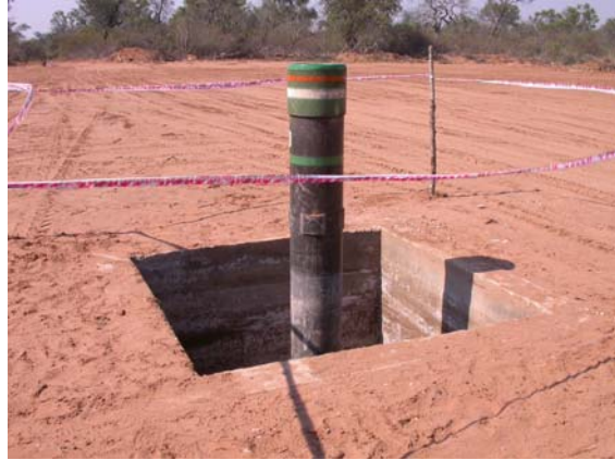
The conductor pipe drilled and cemented 50 meters into the ground and the 2m deep drill cellar ready for the drill rig to set up at the twin well to the Independencia 1 well
